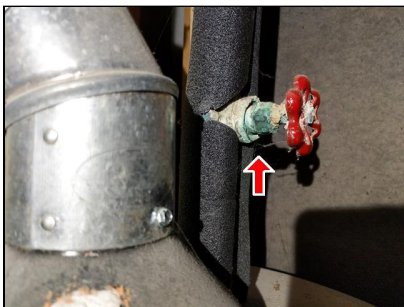
8.1 Item 2(Picture) Prior leak at shut-off valve over water heater
