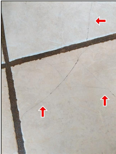
4.2 Item 1(Picture) Floor tiles damaged
