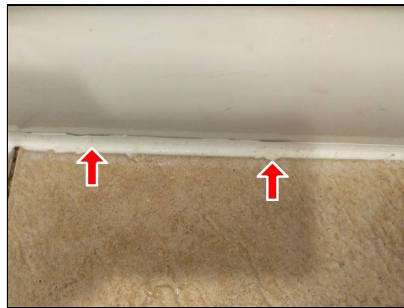
6.7 Item 3(Picture) Seal deteriorating
