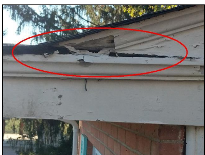
2.5 Item 2(Picture) Gap in wood trim over front porch
