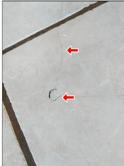
4.2 Item 2(Picture) Floor tiles damaged
