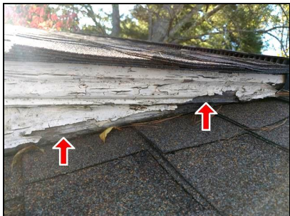
2.5 Item 3(Picture) Paint peeling on trim
