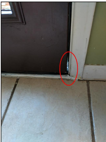
4.3 Item 1(Picture) Gap at bottom of door when closed
