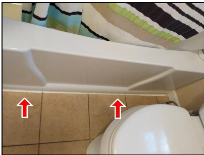
6.7 Item 2(Picture) Seal deteriorating at floor
