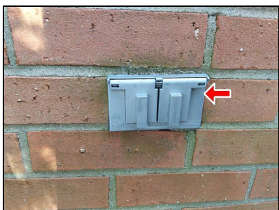
2.7 Item 1(Picture) Outlet not GFCI protected
