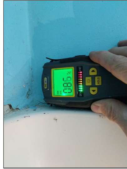
6.1 Item 3(Picture) Moisture meter reading
