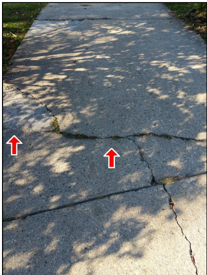
2.4 Item 1(Picture) Driveway damaged
