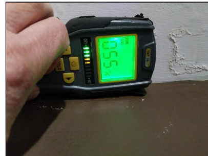
5.0 Item 3(Picture) Moisture meter reading
