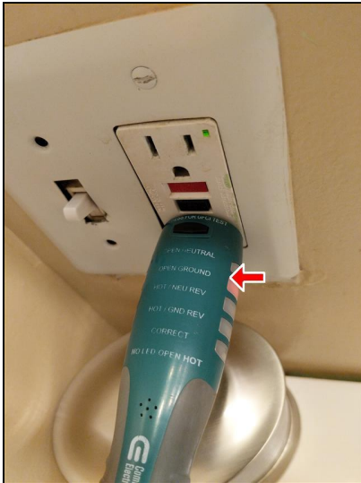
6.8 Item 1(Picture) GFCI outlet not grounded
