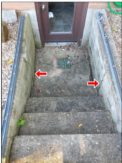
2.3 Item 3(Picture) Retaining walls damaged
