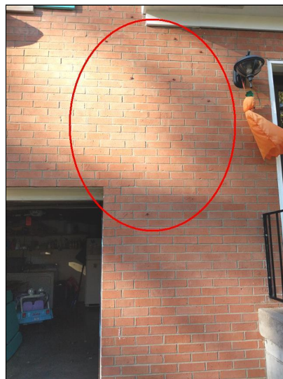
2.0 Item 2(Picture) Location of crack
