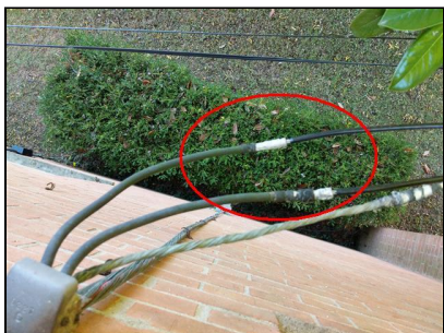
9.1 Item 3(Picture) Insulators missing
