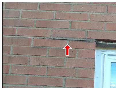
2.0 Item 6(Picture) Mortar deteriorating on right side
