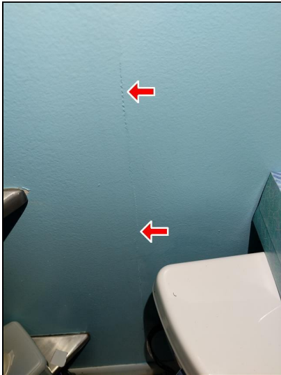
6.1 Item 5(Picture) Crack in wall behind toilet
