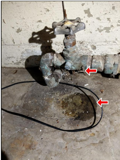
8.1 Item 1(Picture) Leak at main water shut-off valve
