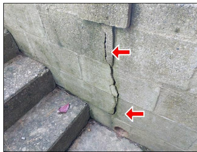
2.3 Item 5(Picture) Crack in wall blocks
