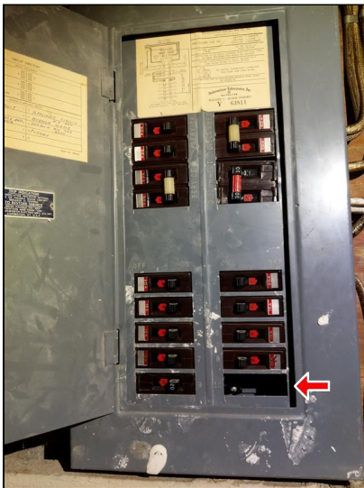
9.1 Item 4(Picture) Knockout cover missing
