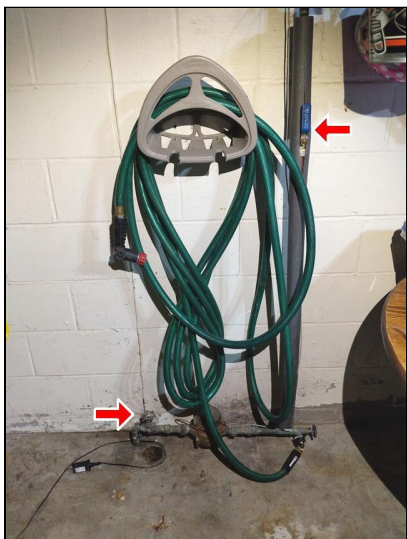
8.3 Item 1(Picture) Main water shut-off
