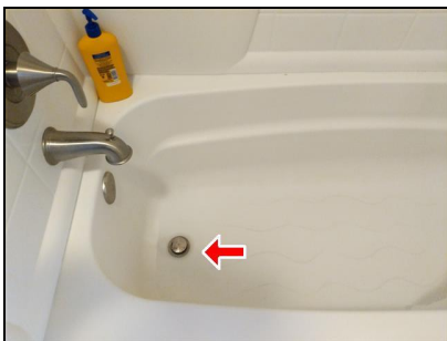
6.6 Item 1(Picture) Bathtub slow to drain
