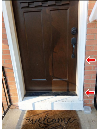
2.1 Item 2(Picture) Location of gap
