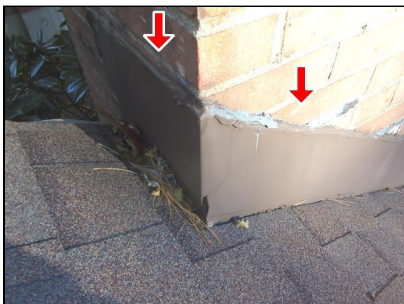
5.0 Item 4(Picture) Seal deteriorating around chimney
