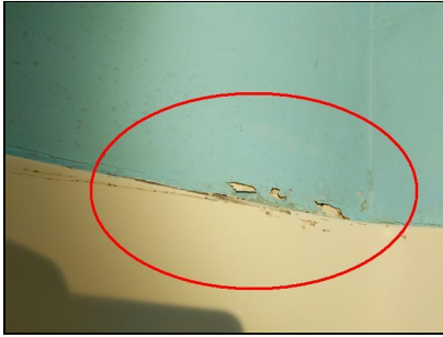
6.1 Item 1(Picture) Moisture damage on wall
