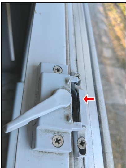
5.5 Item 1(Picture) Window in master bedroom will not lock properly
