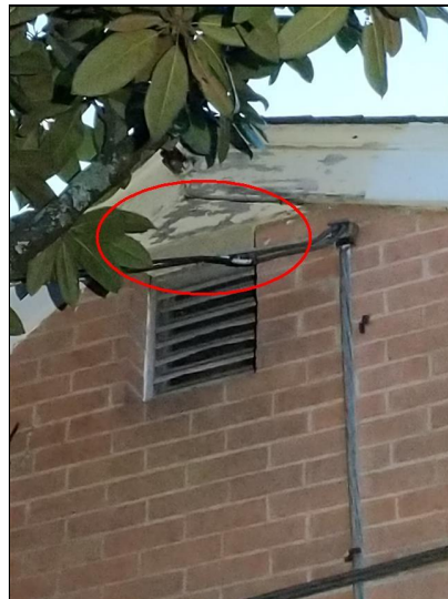
1.5 Item 2(Picture) Location of gap
