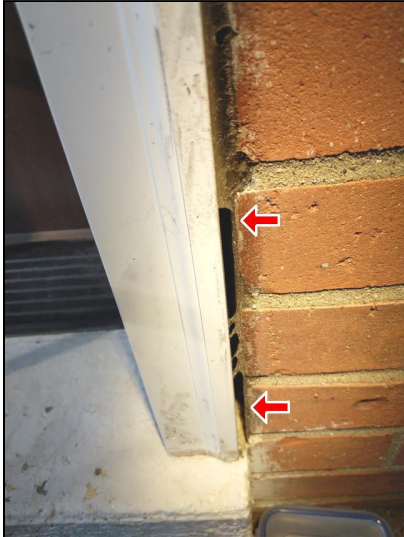
2.1 Item 1(Picture) Gap at door frame, front of house
