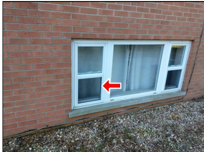
2.2 Item 2(Picture) Location of damaged window
