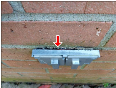
6.1 Item 4(Picture) Source of moisture intrusion
