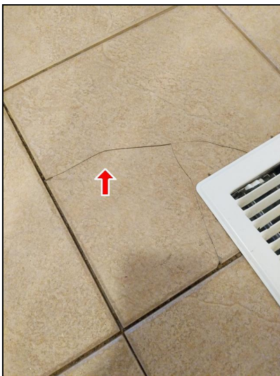
6.2 Item 1(Picture) Floor tiles damaged
