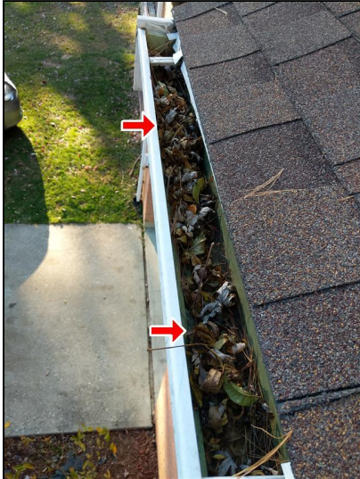
1.4 Item 1(Picture) Debris in gutter
