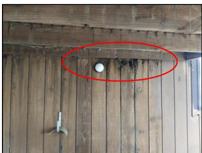
2.3 Item 9(Picture) Wood rot on siding under deck
