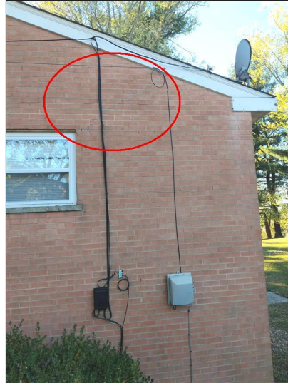
2.0 Item 4(Picture) Location of crack
