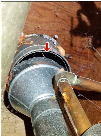
8.2 Item 2(Picture) Vent not properly connected
