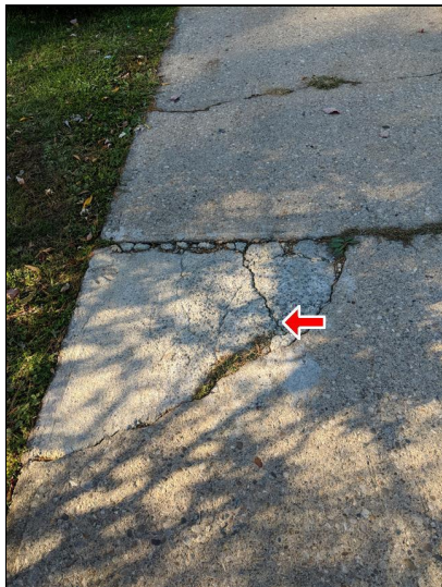
2.4 Item 2(Picture) Driveway damaged
