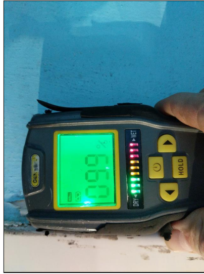
6.1 Item 2(Picture) Moisture meter reading
