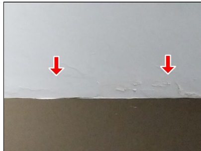
5.0 Item 2(Picture) Moisture staining on ceiling
