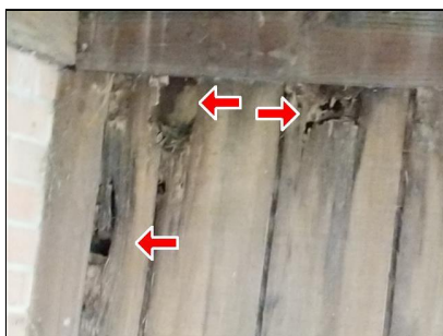
2.3 Item 10(Picture) Wood rot on siding
