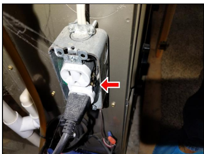
10.1 Item 1(Picture) Cover plate missing
