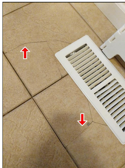
6.2 Item 2(Picture) Floor tiles damaged
