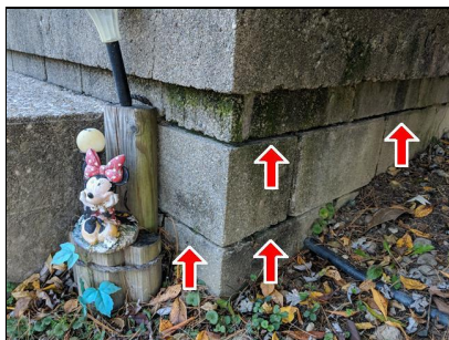
2.3 Item 2(Picture) Gaps in mortar at front porch
