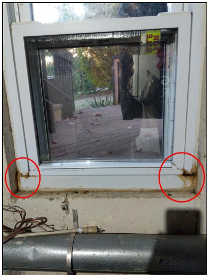
3.4 Item 1(Picture) Signs of moisture intrusion at garage window
