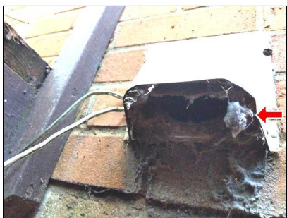
2.8 Item 1(Picture) Dryer vent needs to be cleaned
