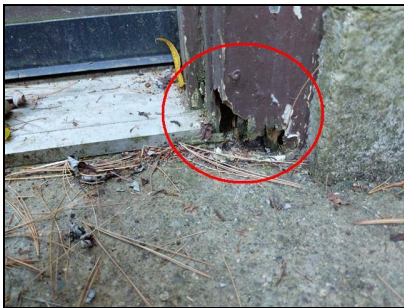
2.1 Item 3(Picture) Wood rot on door framing, rear of house
