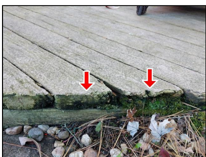
2.3 Item 7(Picture) Deck boards deteriorating
