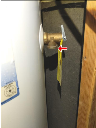
8.2 Item 1(Picture) T&P pipe missing
