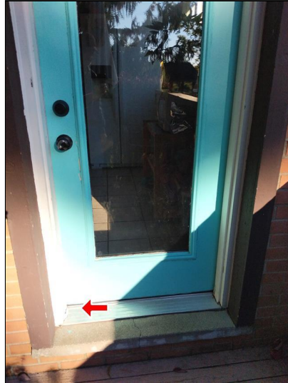
2.1 Item 6(Picture) Location of wood rot
