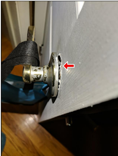
5.4 Item 1(Picture) Door handle loose, hallway closet
