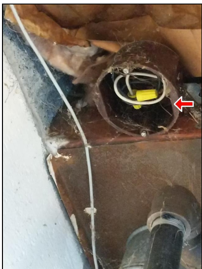
3.7 Item 1(Picture) Cover plate missing
