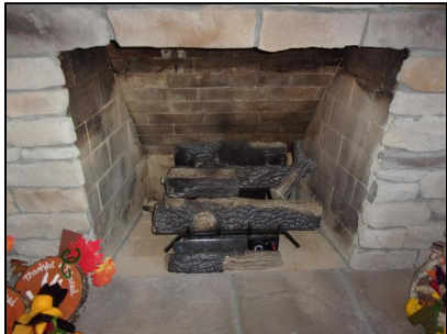
10.6 Item 1(Picture) Gas fireplace
