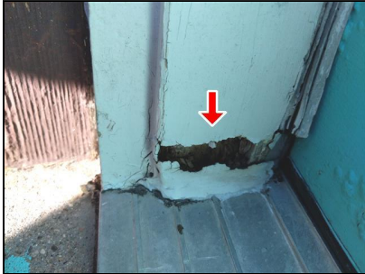
2.1 Item 5(Picture) Wood rot on door framing
