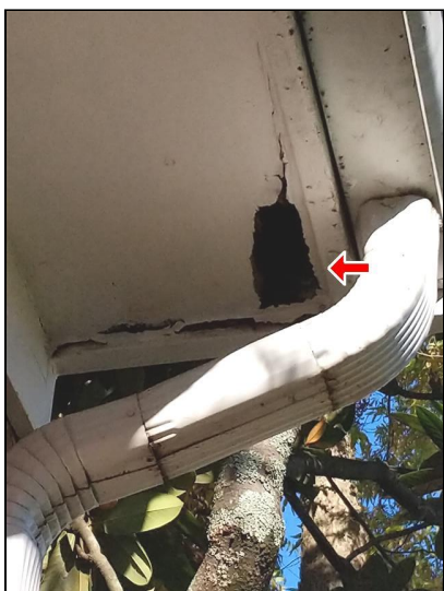
2.5 Item 1(Picture) Hole in soffit panel, right front
